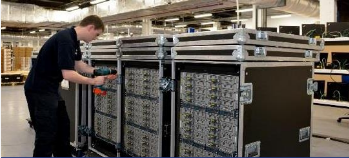
Data Center and network deployment
